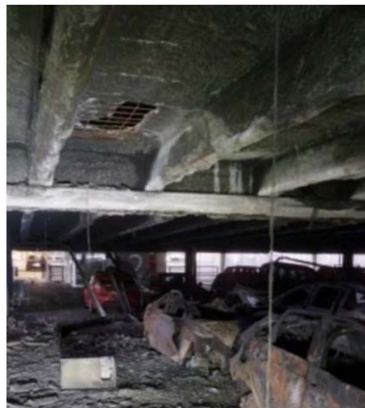
Stavanger Norway 2020. Concrete spalling example. NFPA Parking Structure Report 2020
