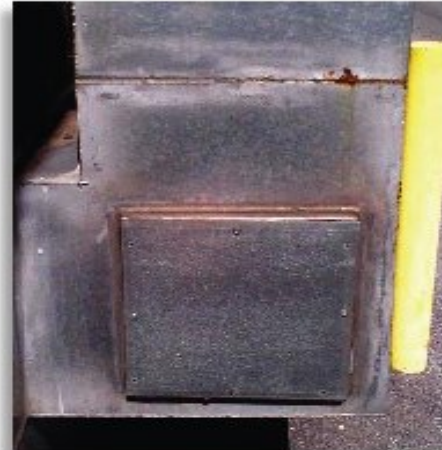
This duct access panel should be fully attached and the corrosion checked for potential failure points.
